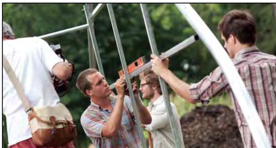
Jeff McCabe has a plan to build 20 hoop houses in the 20 days leading up to July 4th, 2011. "Scheduling to build them by the 4th of July was intentional. It's a good time of the year to celebrate, but also it's a good time for the farmers to have the hoop houses and start using them."
